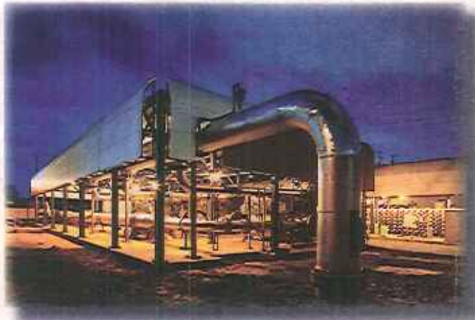
Photo courtesy of West Basin Municipal Water District
